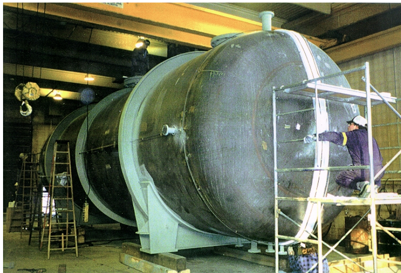
Figure 2.2 While the insulation being applied to this pressure vessel is not within the scope of Division 1, the insulation anchors welded to the vessel shell and head must meet Division 1 requirements (UG-55).
